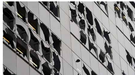
GLASS WINDOW DAMAGE FROM HURRICANE
